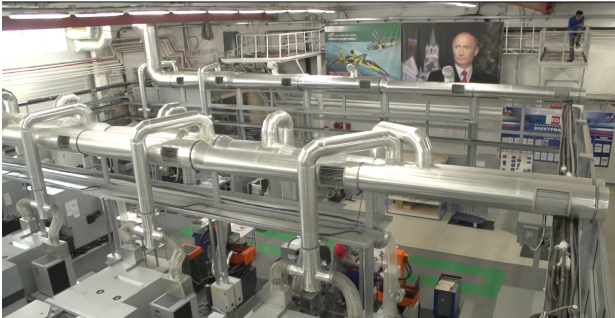
Figure 4: KZE Production Facility in Karachevsk
